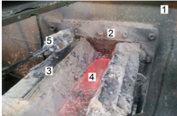
Tap hole in the mixer wall
